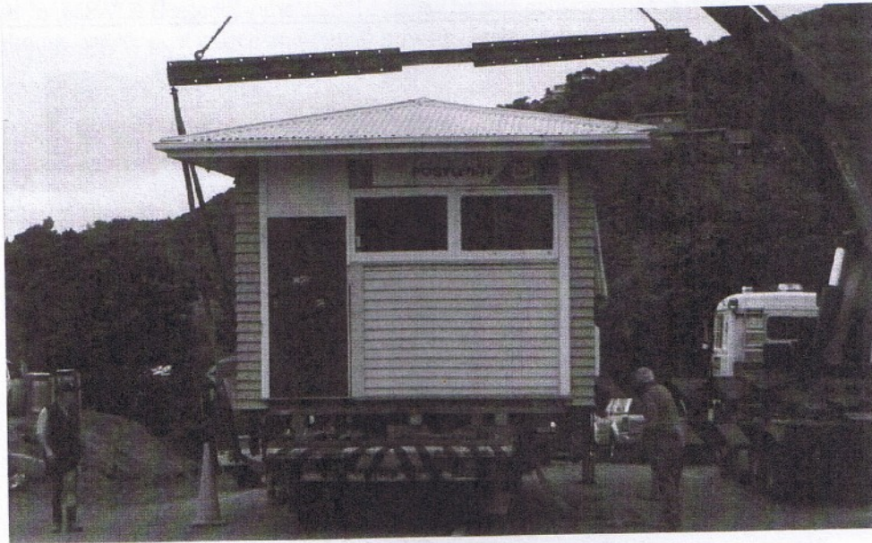
On the move again. Transfer of the Piha PostCentre to its new permanent site in the Domain on 12 October 2009 [photo: ex Coney (2008-10)].
